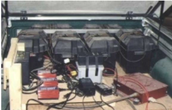
Fig. 7. Power supply and regulation system (see Table 4) in place on the deck
