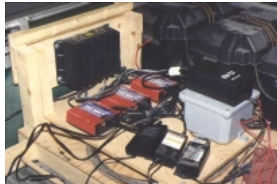
Fig. 8. Battery charger (left), converters (red) for DC to AC conversion and inverters (black) to convert AC to DC for instruments and notebook computers
